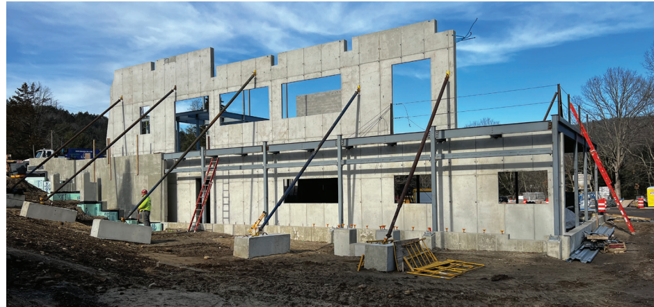
The designers for the DEEP project designed a thermal mass wall utilizing concrete made with post-consumer ground-glass pozzolan cement to optimize the site's solar orientation all year round. The Trombe wall provides passive heating and cooling and improves natural ventilation.
