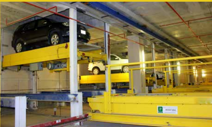
Start up and testing is done before the garage is turned over to the owner.
