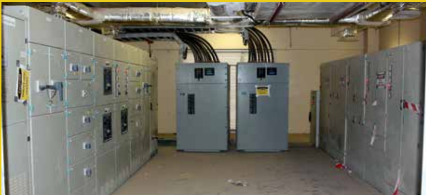
This is the electrical room for the system.
