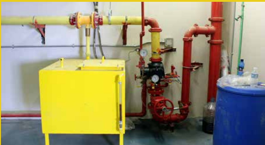
This is a portion of the fire-prevention system.
