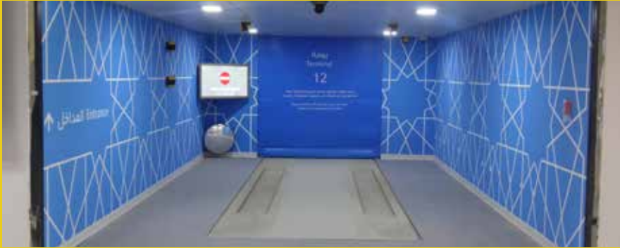
The entry/exit terminals are the only part of the system that the user encounters. A luxurious setting provides for an upscale user experience.
