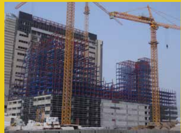
The steel framing is erected. In this development, conventional parking is on the bottom, with the APS above it.
