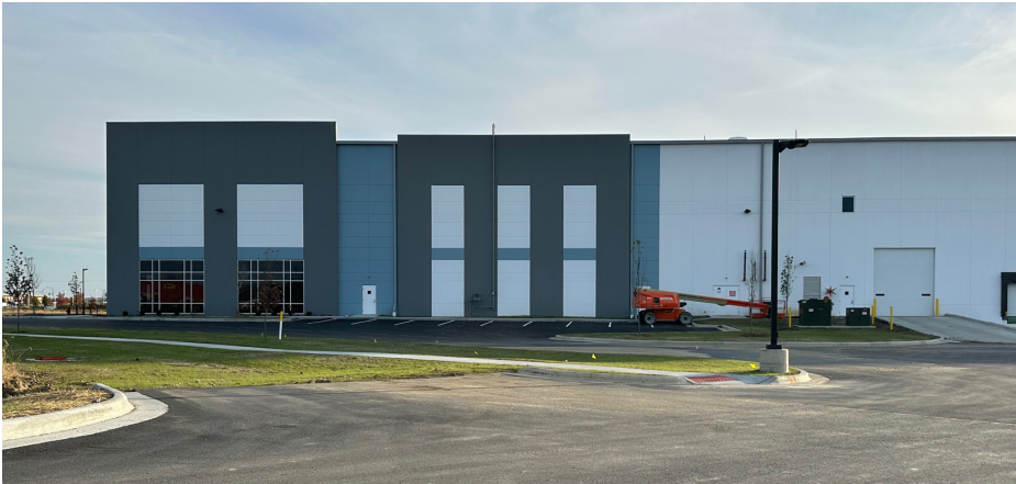
This concrete tilt-up building was limited to solid colors. The paint has no long-term warranties.
