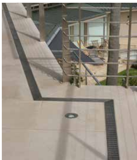
Balconies require management of water, too, which can be provided, as shown above, with a continuous linear drain near the edge to collect and remove water.
