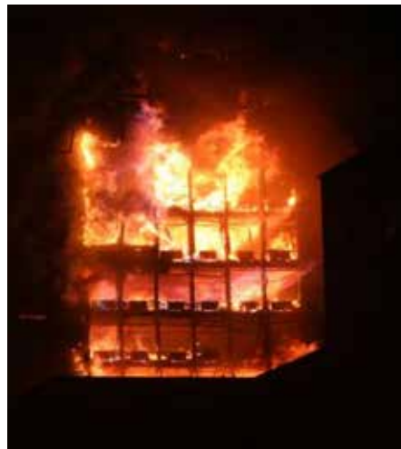
Notice the flame height attacking the exterior on The Windsor high-rise in Madrid, Spain, that was destroyed by fire in 2005.
