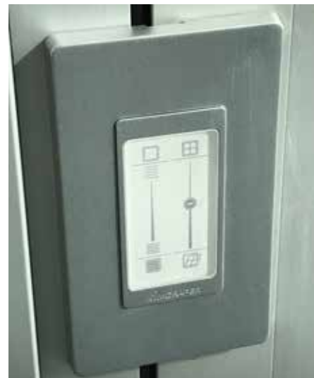
Exterior shading with an integrated control system helped DIALOG deliver a net-zero design for the University of Calgary's MacKimmie Tower.
