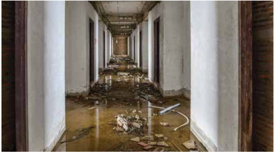
An undetected water leak can cause considerable damage to a building, interrupt building operations, and create potentially unsafe indoor environments for occupants.
