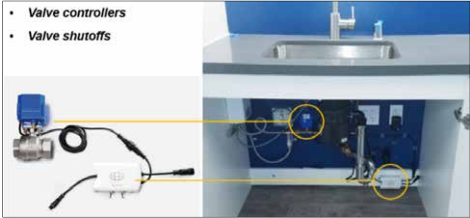
Electronically controlled valve controllers and valve shut-offs are an integral part of a complete, effective, wireless water leak detection system.
