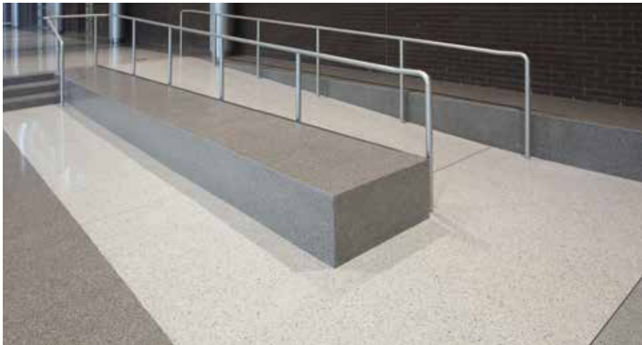
A patterned epoxy terrazzo floor with short walls, 20-foot-long tread and risers, and a handicapped-accessible ramp lend durability and aesthetics to Eureka High School’s new STEM addition in Eureka, Mo.
