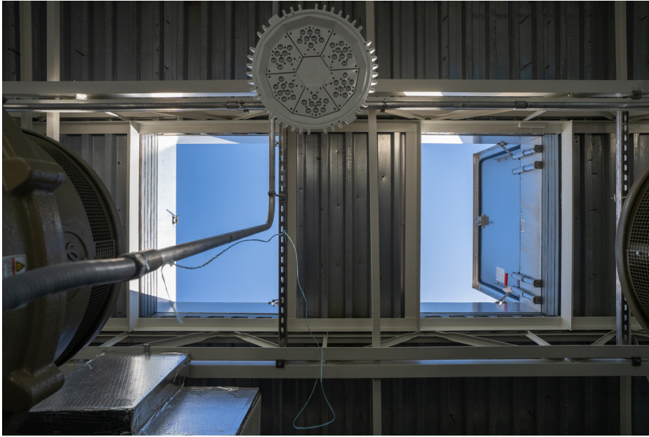
Ten roof hatches at a reclamation facility in Parker, Colorado, provide workers with access to equipment for maintenance and replacement purposes.
