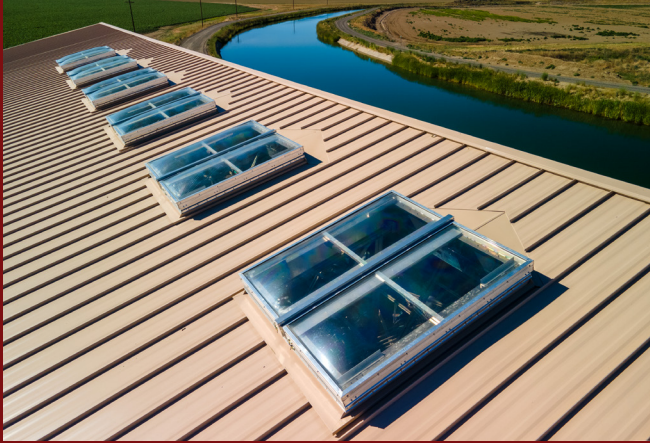
Roof hatches are critical to a pumping station that refills an aquifer.
