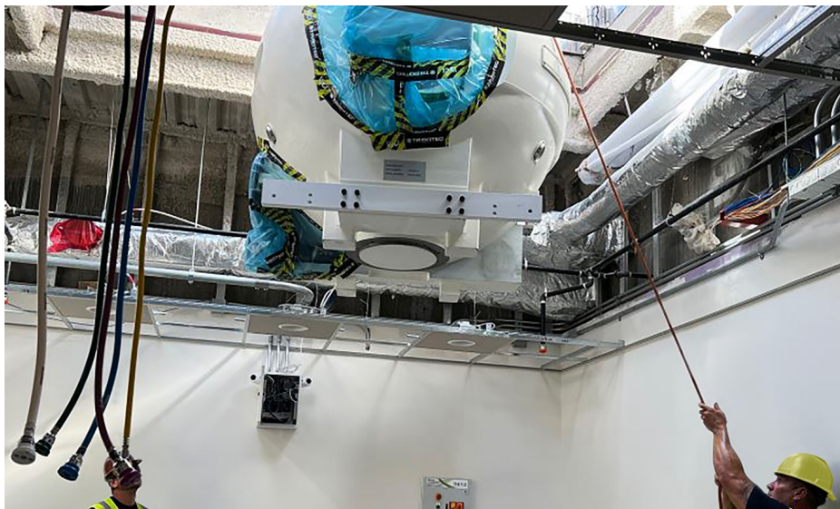
A large roof hatch allows this massive Gamma Knife unit to be lowered into an oncology suite at Ochsner Medical Center in New Orleans.
