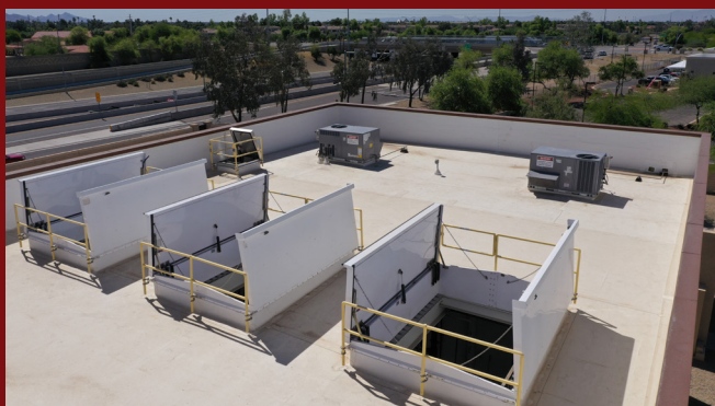
Hatches with safety rails were critical to this water reclamation facility in Glendale, Arizona.
